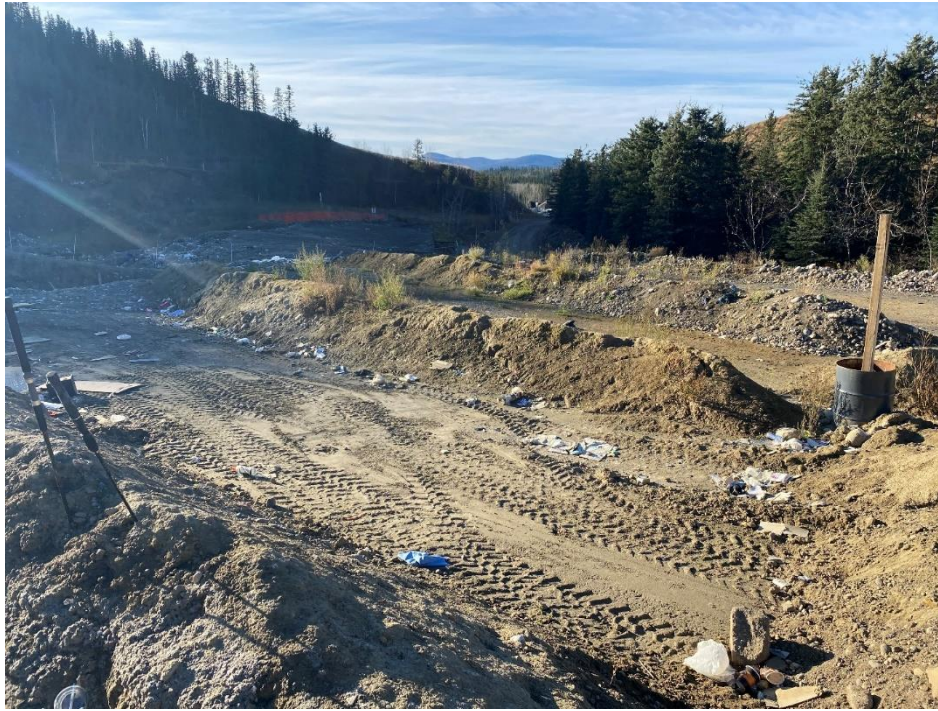
Photo 2: Litter Containment Berms used to contain refuse at Carmacks
