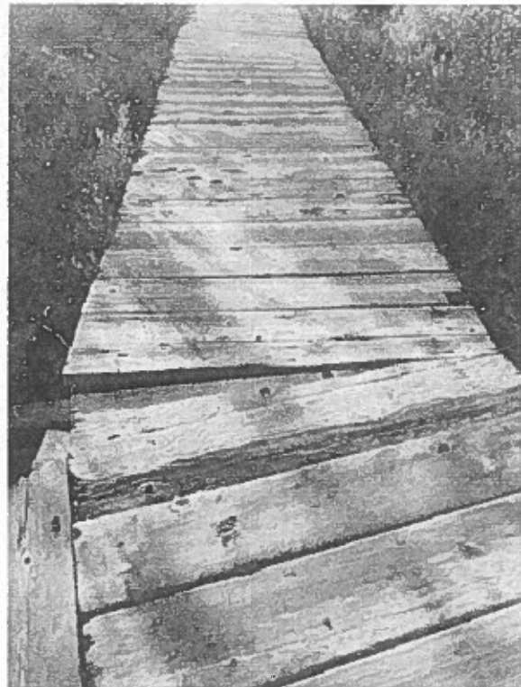
Typical current tripping hazards.
